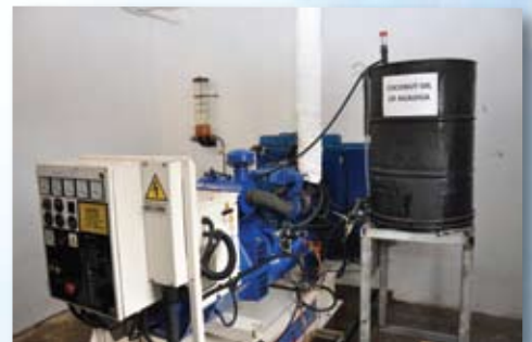
Picture 3: Generator running on Coconut Oil
